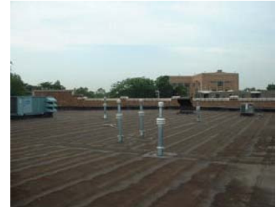
The existing un-coated modified bitumen roof has aged prematurely and appears brown because of the oils that have "cooked out" of the membrane.
