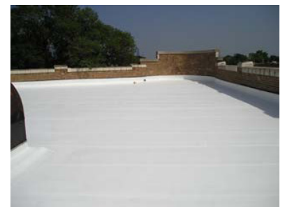
After coating with Lucas #1000TC, the same roof is sealed and protected with a cool white finish that will reflect heat and prolong the roof's service life.
