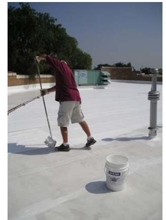
Lucas #1000TC is applied over a base coating of Lucas #1000MB. Lucas base coatings are specifically designed for maximum adhesion to different types of roof systems.
